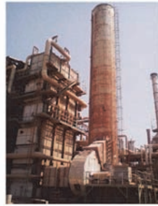
Reformer (Exhaust Dust)
