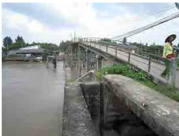
One of the potential sites where sluice gate is to be installed. The sluice gate together with others is to prevent saline intrusion to the coastal areas.
