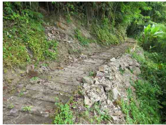
Photo 1-6 Wooden cover which was set up by collapse from jointed bedrock to keep the headrace structure
