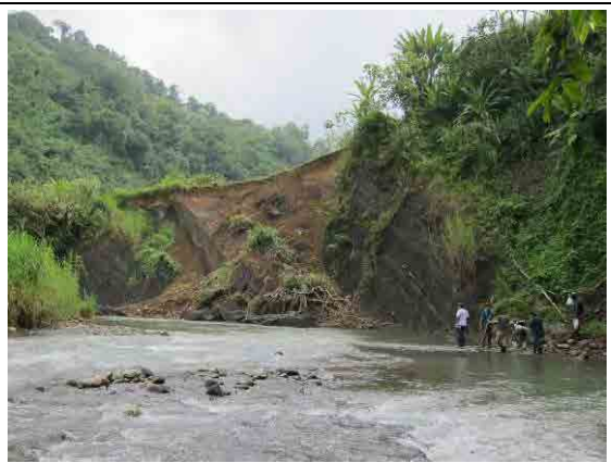
Photo 1-8 (after collapsed ; October) same part as left Collapse of the central portion was occurred caused by water penetration after heavy rain
