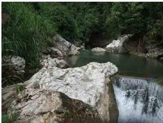
Photograph 3: Current conditions of irrigation water intake weir. Currently, the river water isn't acquired but simply flows over the weir. In the Project, it is planned to rehabilitate this weir (raising by approximately 0.3 m) with a view to in-taking a maximum of 2.0\text{m}^3/\text{s} of water.
