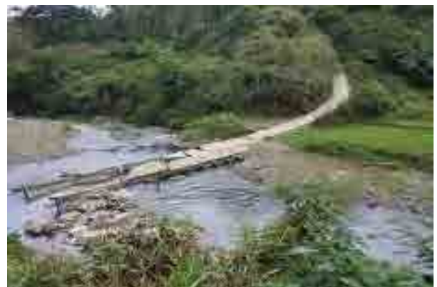
Washed out bridge
