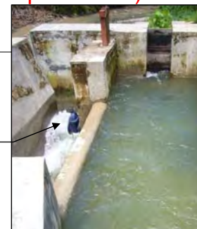
Water Diversion for Irrigation System
