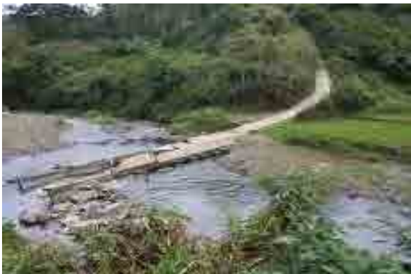
Washed out bridge
