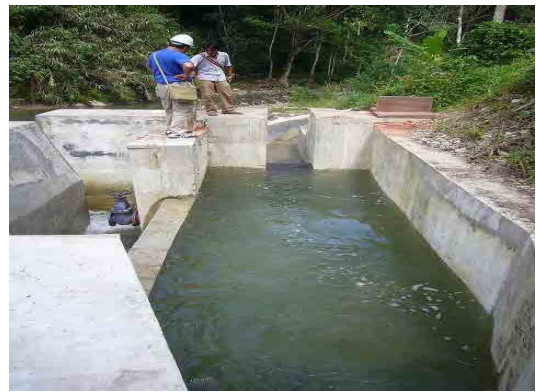
Plate 2-2 Settling and Basin 1
