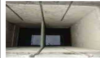
Vertical Baffle type Flocculator
