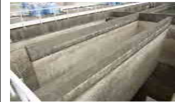
Horizontal Baffle type Flocculator
