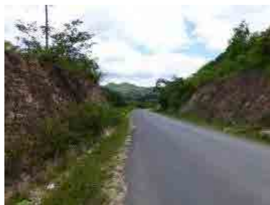
Photo 2-2-3 Excavated Slope Condition along Major Road
