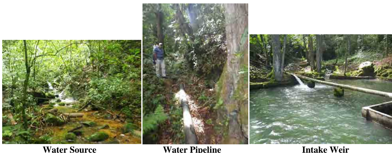
Photo 1-3-7 Water Source, Pipeline and Intake Weir of Picacho Water Treatment Plant
