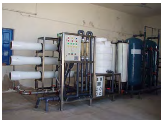
写真 5.2-1 Existing RO Plant (#4)
