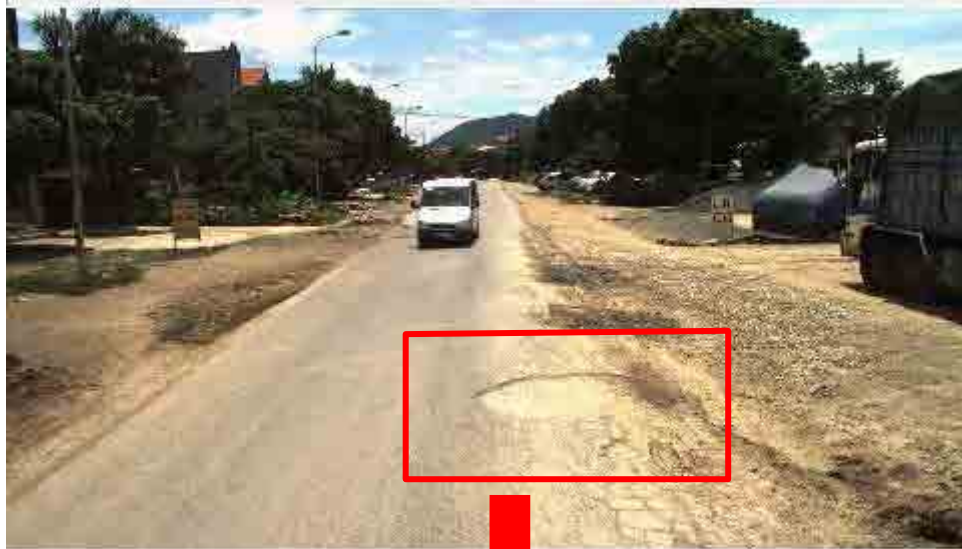
Figure 4.37 Pothole - Front View,
