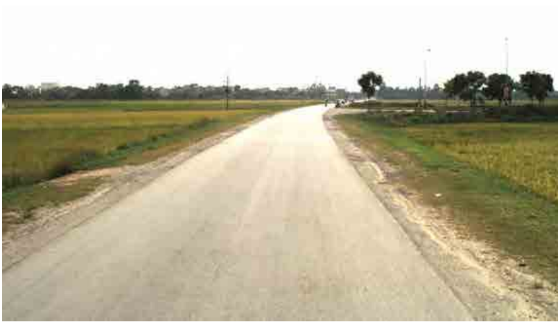
Figure 42 Crack Ratio 10% (Outbound NH.38, 15k100-15k200)
