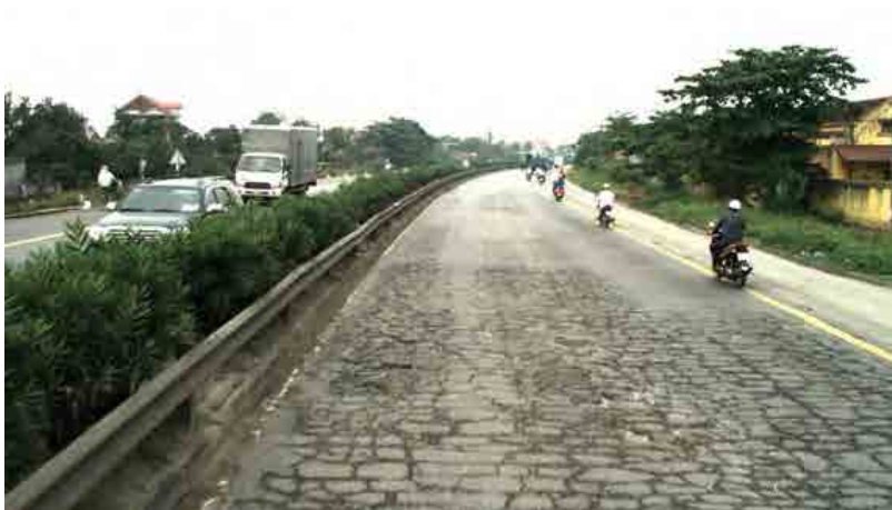
Figure 44 Crack Ratio 70% (Inbound NH.5, 84k000-84k100)
