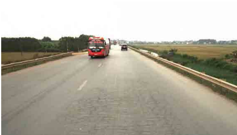
Figure 43 Crack Ratio 30% (Inbound NH.18, 17k200-17k300)
