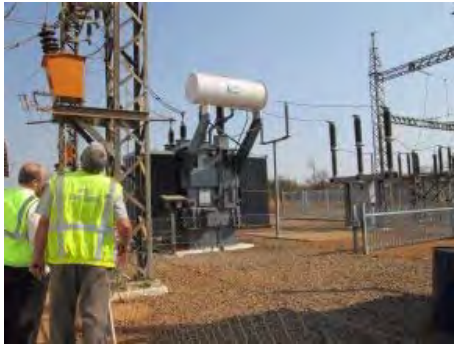
(a) Transformer for AC Substation
