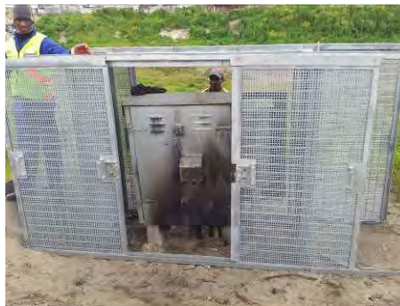
Source: Photo taken by Study Team Figure 4-9 Theft Prevention Measure
