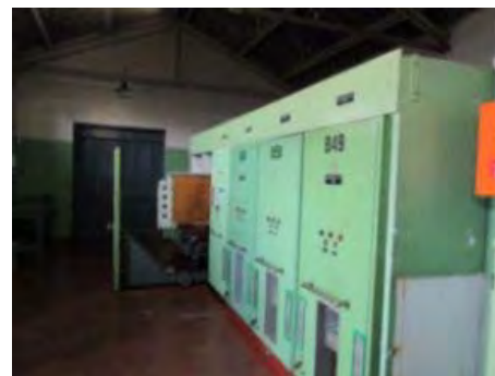
(b) High-speed Open Air-type DC Circuit Breaker (HSCB)
