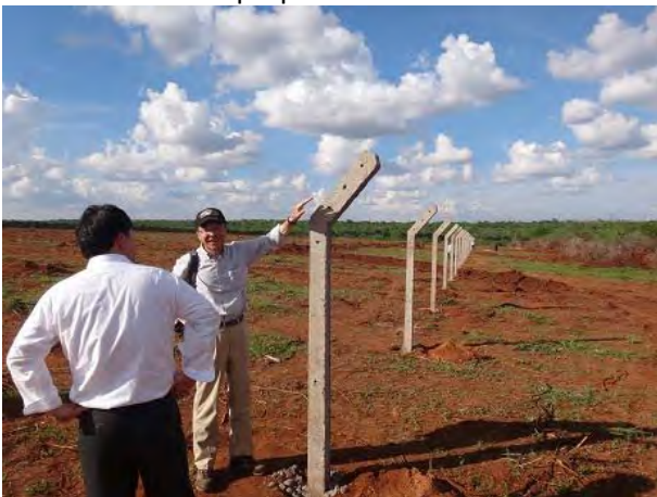
Fencing by concrete pole with barbed wire
