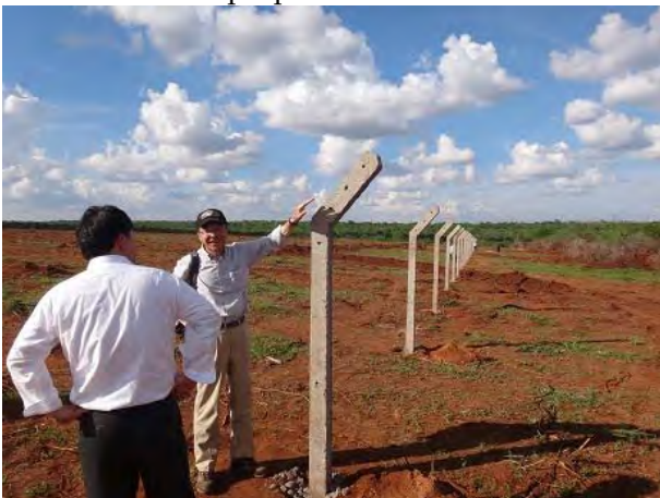
Fencing by concrete pole with barbed wire
