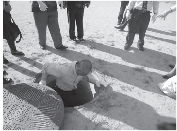
1/10 Storm Overflow Chamber at Kimachi Park
