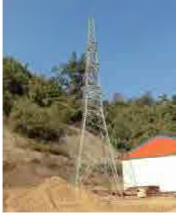
Transmission line facilities
