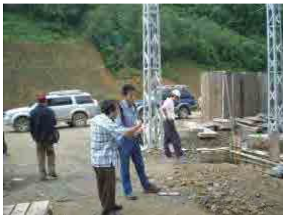
OJT at switchyard
