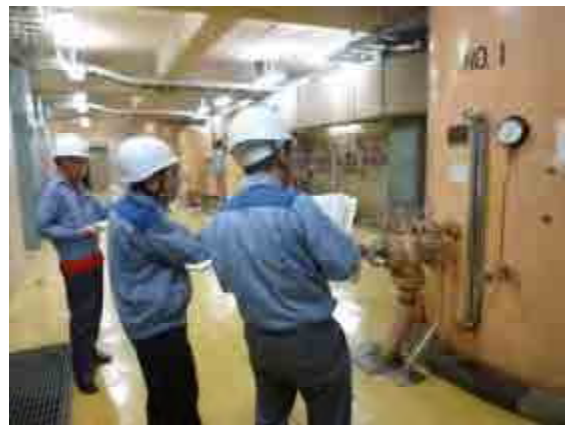
OJT (Amagase Hydropower station)
