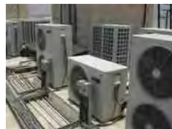
Outside units on rooftop
