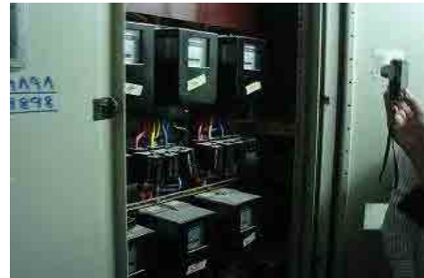
(b) Electricity Meters in Building for Rent
