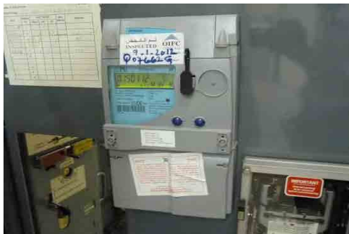
(a) Digital Meter with Communications for High Voltage Customers
