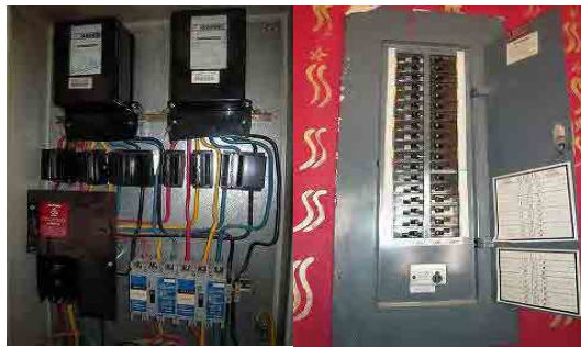
(a) Residential Electricity Meter and Distribution Board
