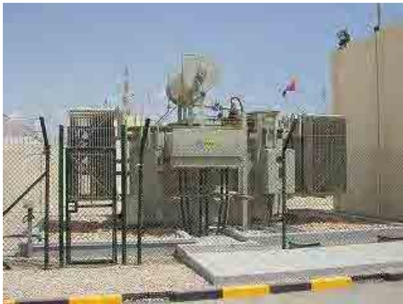
(c) 33/11 kV Transformer
