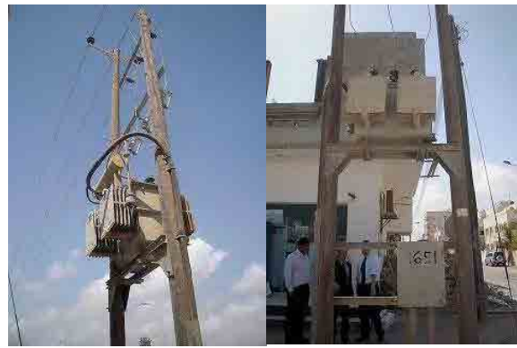
(b) Pole-Mounted (315 kVA)
