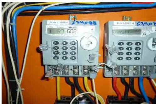
(a) Prepaid Meter in Electrical Room
