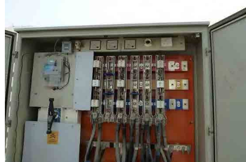
(b) Digital Meter with Communications at the secondary side of DSS
