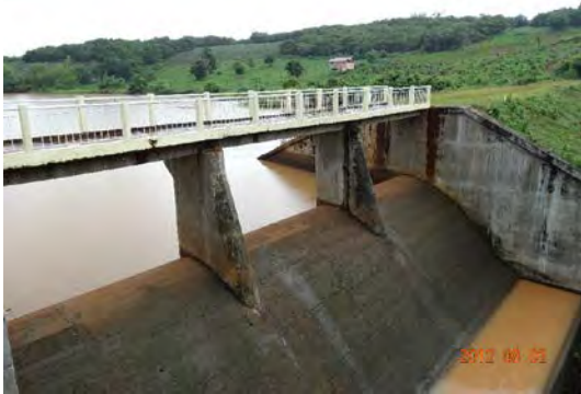
(8) Spillway of O'Chum No.2 Dam: Though nearly 20 years old, its structural integrity has not been compromised.
