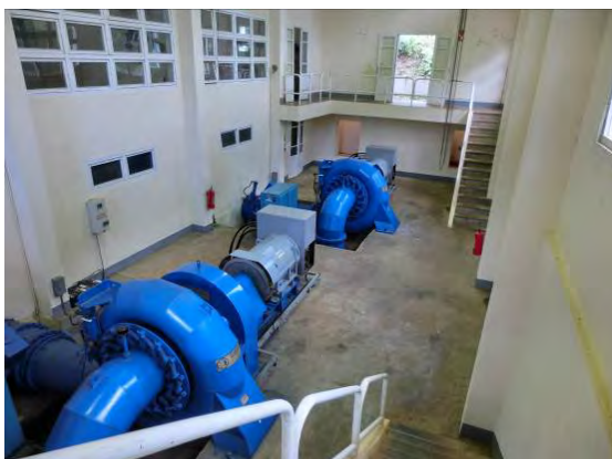
(10) O'Chum No.2 Power Station, whole view of turbines and generators: The near side is Unit No.2, and the far side is Unit No.1. Operators work in 3 shifts, 1 in each shift and 4 during the day shift, to generate power.
