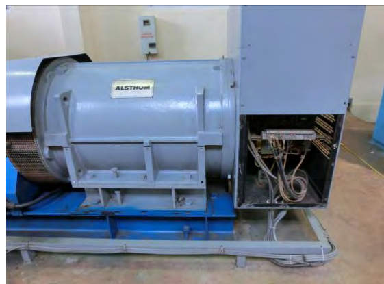
(11) O'Chum No.2 Power Station, condition of generator: The exciter is severely deteriorated due to aging. Turbine has cavitation and is worn out.
