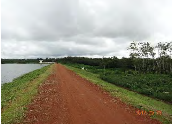
(6) Dam crest road: Not open to general vehicles, but used by motorcyclists and pedestrians as a community road.
