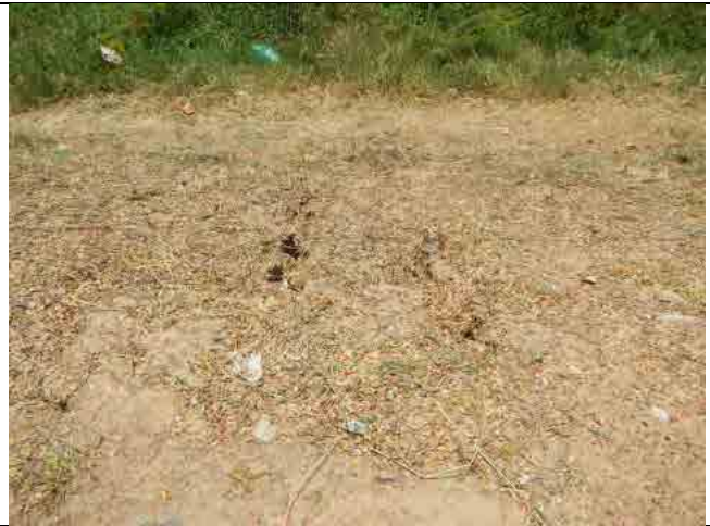
Photo-74: Sec. 23-4, 5 Gully erosion of Top Soil
