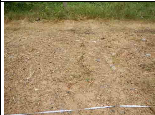
Photo-47: Sec. 16-3 Gully erosion of Top Soil
