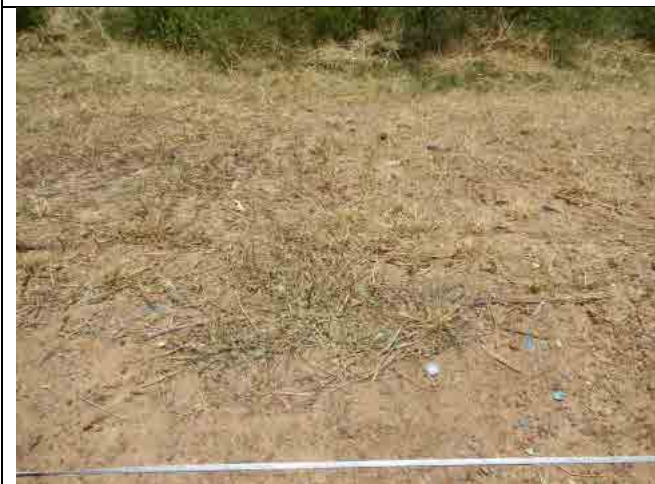
Photo-39: Sec. 14-1 Gully erosion of Top Soil
