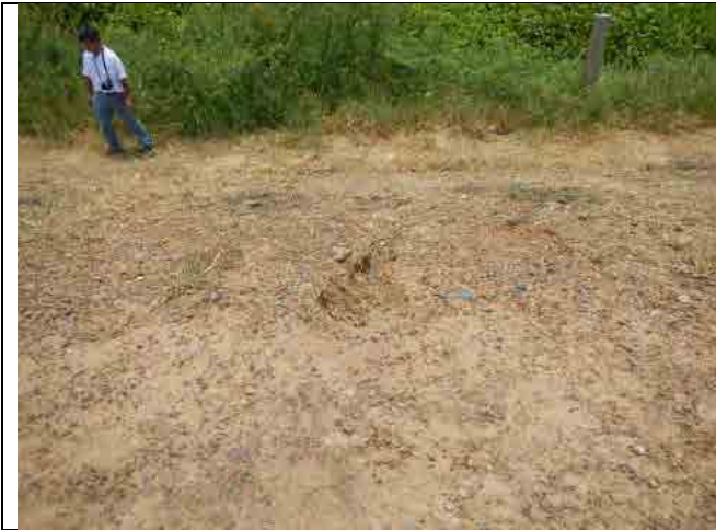
Photo-49: Sec. 17-2 Gully erosion of Top Soil
