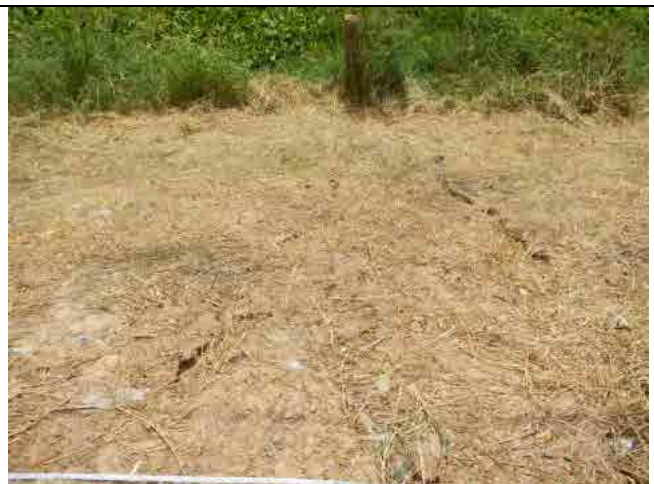
Photo-36: Sec. 13-1 Gully erosion of Top Soil
