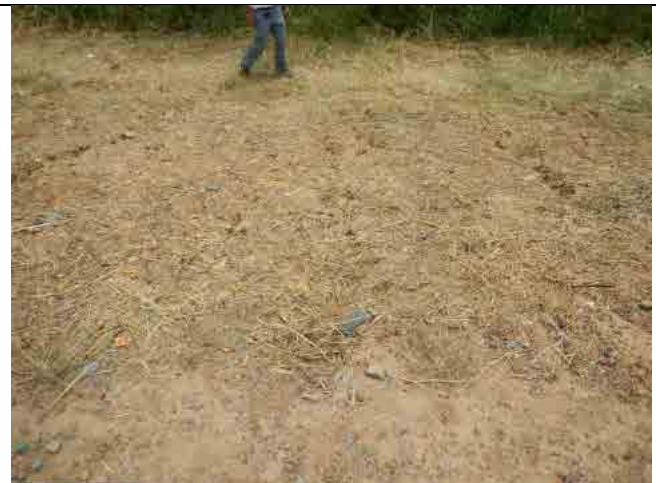
Photo-20: Sec. 8-2 Gully erosion of Top Soil
