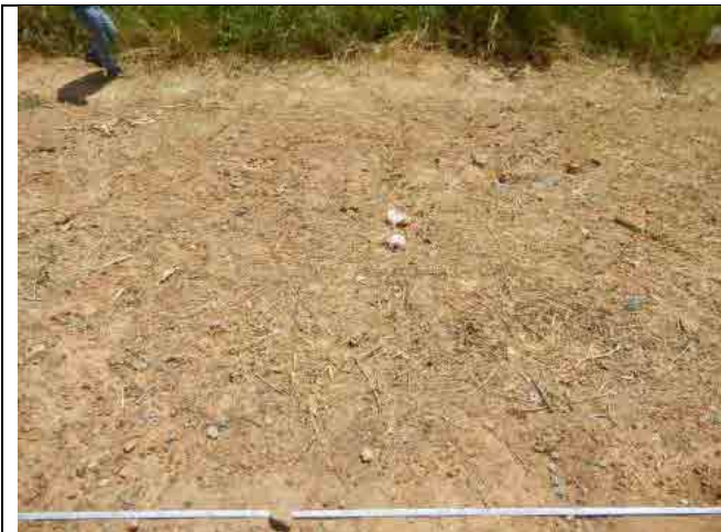
Photo-7: Sec. 3-5 Gully erosion of Top Soil
