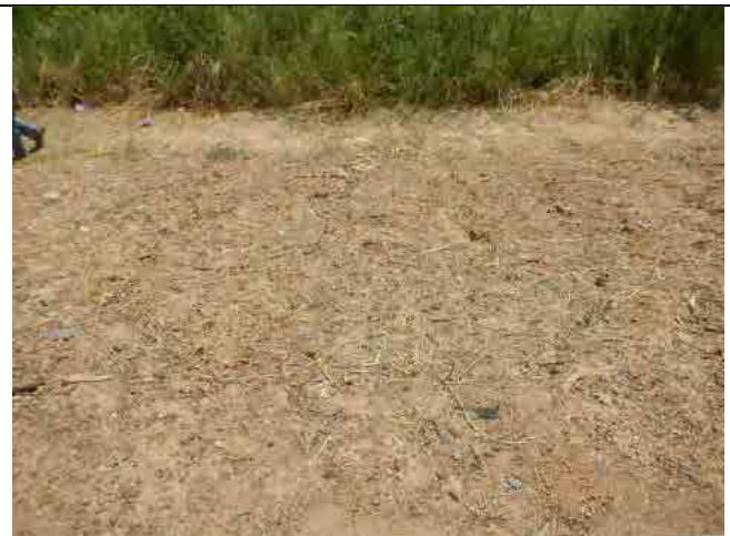
Photo-8: Sec. 4-1, 2 Gully erosion of Top Soil
