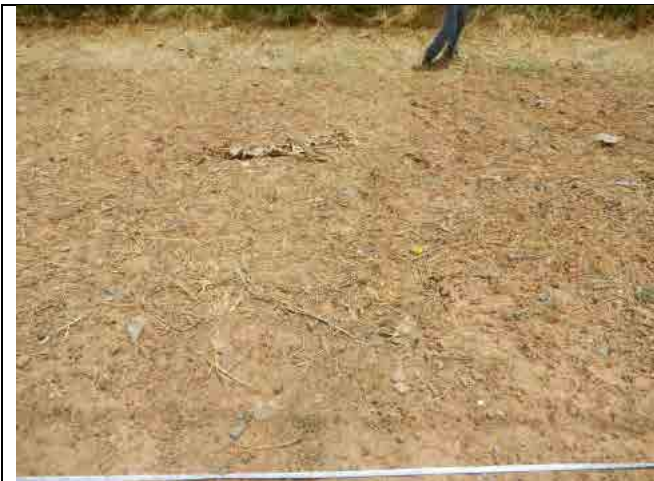
Photo-13: Sec. 5-4 Gully erosion of Top Soil
