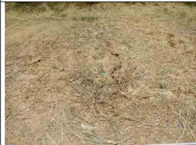
Photo-41: Sec. 14-3, DH Gully erosion of Top Soil and Dragon Hole
