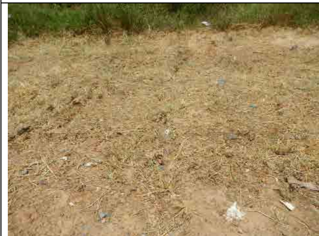
Photo-59: Sec. 19-4 Gully erosion of Top Soil
