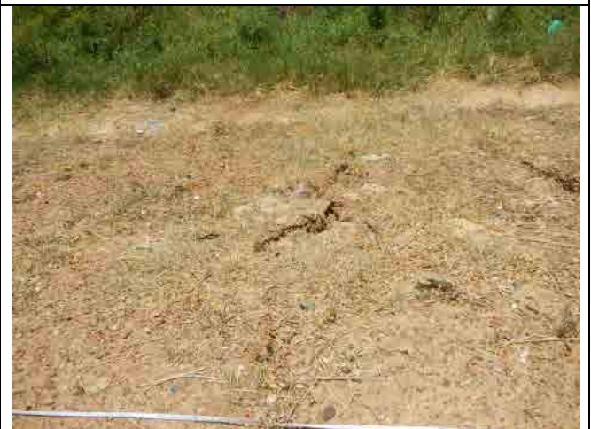
Photo-66: Sec. 21-3 Gully erosion of Top Soil
