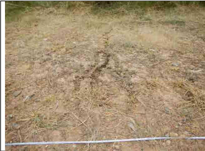
Photo-43: Sec. 15-1 Gully erosion of Top Soil
