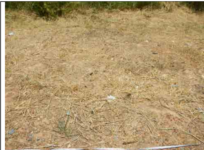
Photo-37: Sec. 13-2 Gully erosion of Top Soil
