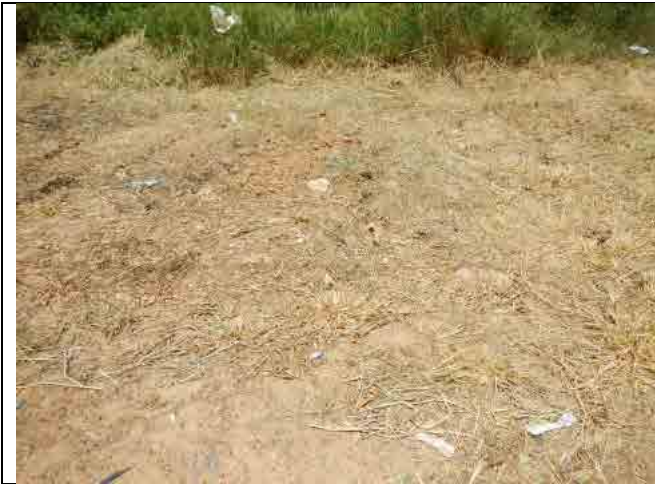
Photo-61: Sec. 20-1 Gully erosion of Top Soil
