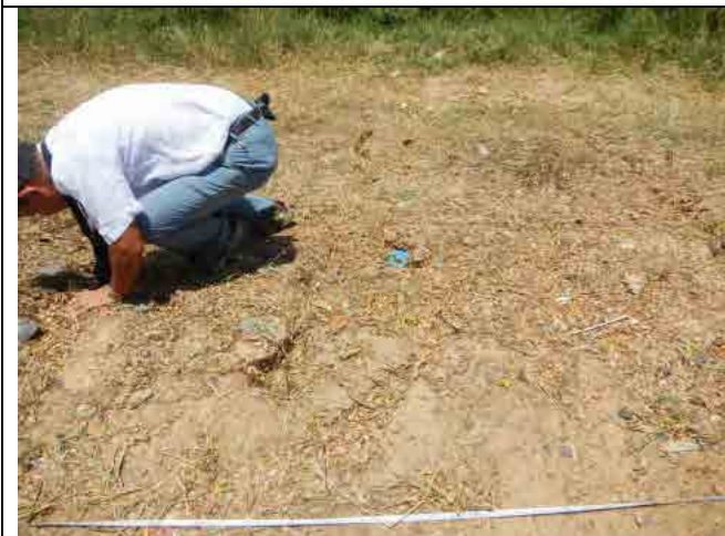
Photo-71: Sec. 23-2 Gully erosion of Top Soil
