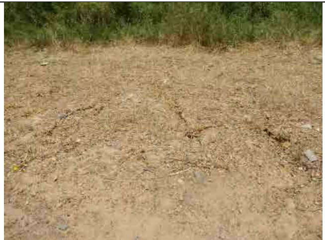
Photo-52: Sec. 18-2, 3 Gully erosion of Top Soil
