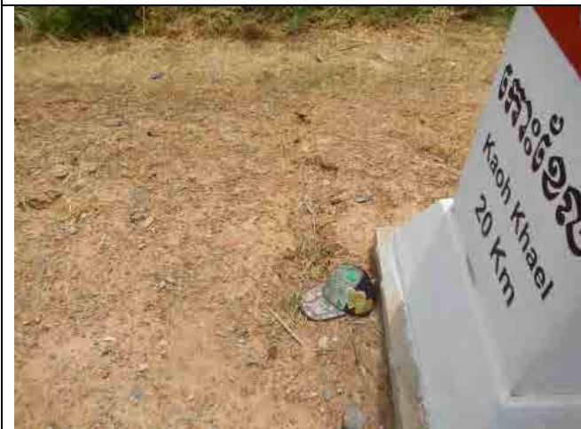
Photo-23: Sec. 9-2 Gully erosion of Top Soil
