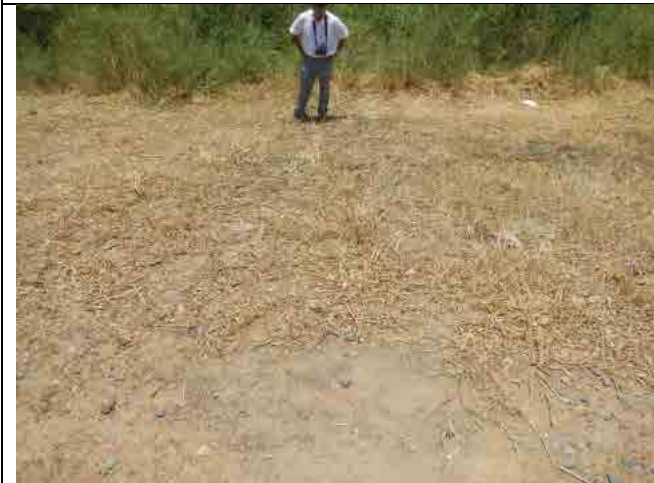
Photo-51: Sec. 18-1 Gully erosion of Top Soil
