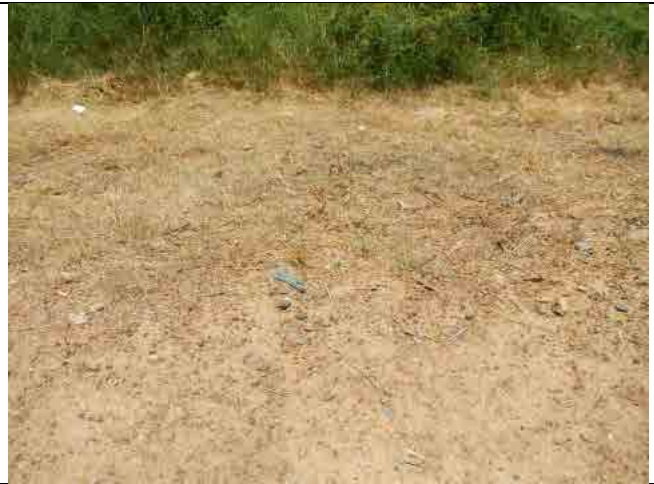
Photo-50: Sec. 17-3 Gully erosion of Top Soil
