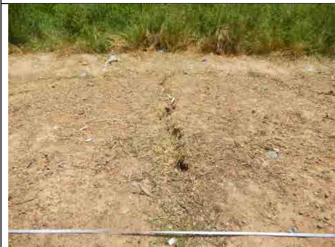
Photo-9: Sec. 4-3 Gully erosion of Top Soil
