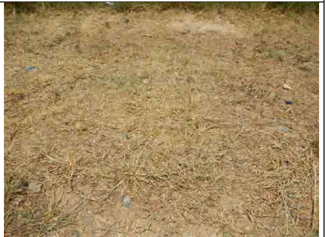
Photo-58: Sec. 19-3 Gully erosion of Top Soil
