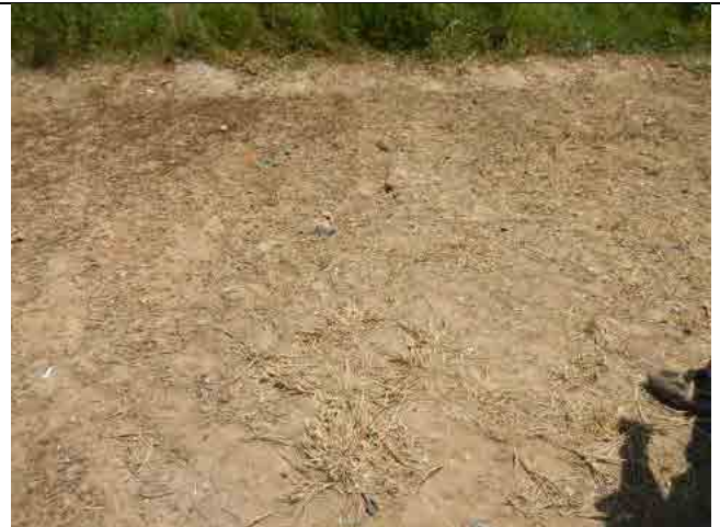
Photo-2: Sec. 1-2 Gully erosion of Top Soil
