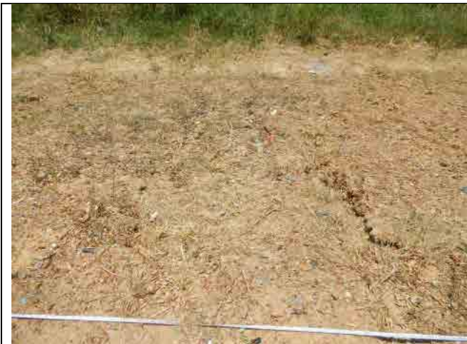
Photo-67: Sec. 22-1, 2, 3 Gully erosion of Top Soil
