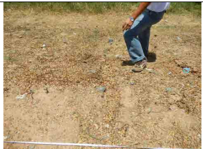
Photo-72: Sec. 23-3 Gully erosion of Top Soil
