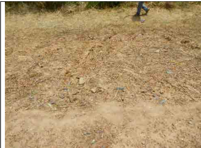
Photo-25: Sec. 9-4, 5 Gully erosion of Top Soil
