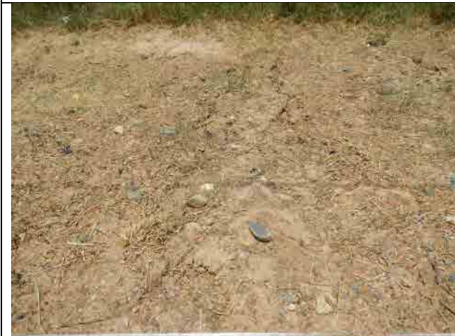
Photo-57: Sec. 19-1, 2 Gully erosion of Top Soil
