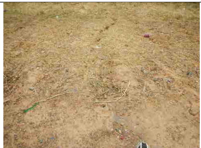
Photo-22: Sec. 9-1 Gully erosion of Top Soil
