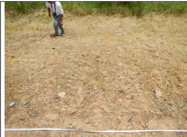
Photo-19: Sec. 8-1 Gully erosion of Top Soil
