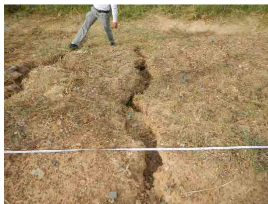
Gully Erosion by Running Water on the Surface of the Slope
