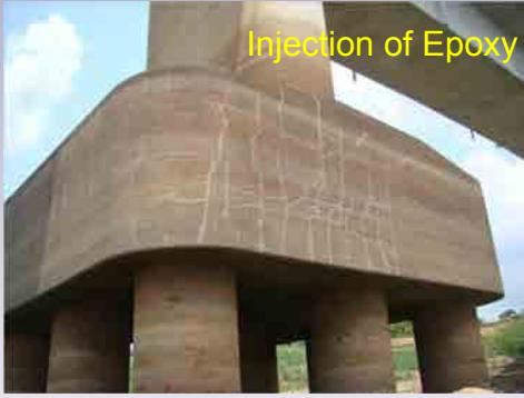
4.Observation (Cracks in P13) Footing (South Side) Latticed Cracks (Vertical, Regular Interval)
