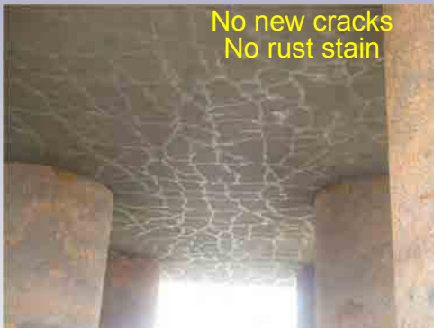
4.Observation (Cracks in P13) Bottom Surface of Footing Radiated Cracks
