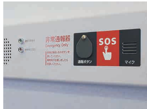
Source: JICA Study Team Figure 3.2.10 Emergency alarm device
