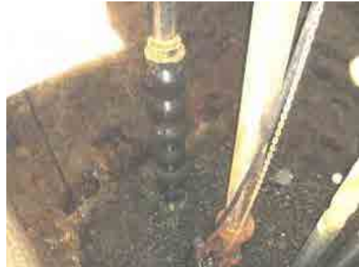
Photo-4 Condition of Intake Well (Shallow Well No.2) of Kampong Cham Waterworks during Dry Season
