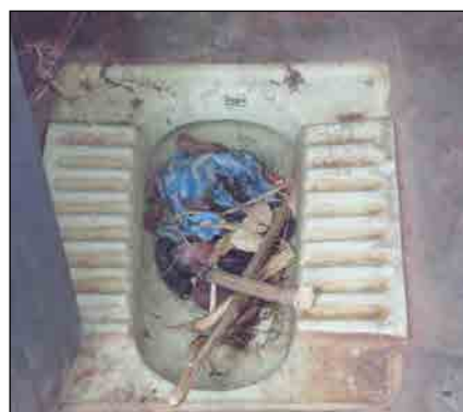
Figure 2.10 Not Used Toilets
