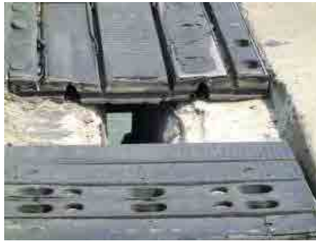
Figure 8.8.2 Deterioration in Expansion Joints
