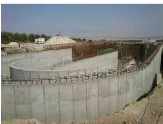
Waste Water Treatment Plant
