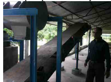
Purified silica conveyer
