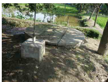
Biogas pipe and digester tank
