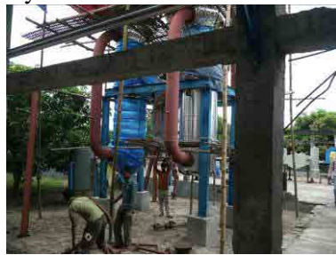
CO2 recovery facility
