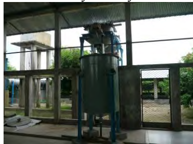
Silica drying facility
