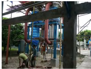
CO2 recovery facility
