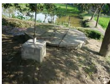
Biogas pipe and digester tank
