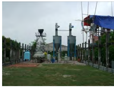
Whole view of the plant
