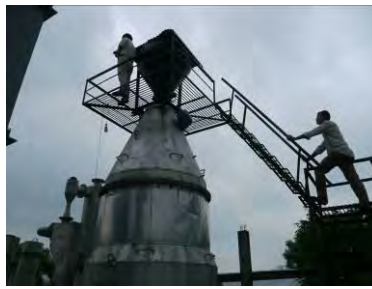
Down draft gasifier
