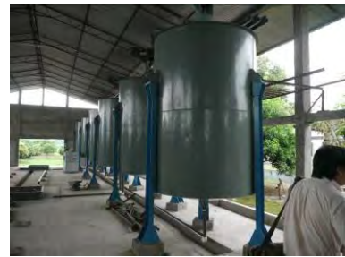
Silica precipitation facility
