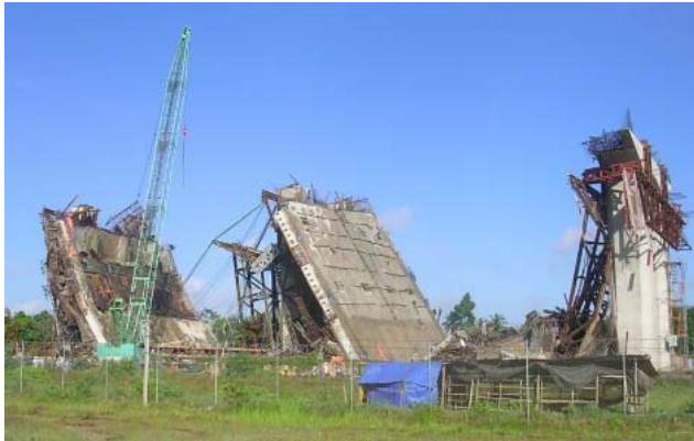
Photo 1 Collapse Accident of Can Tho Bridge in 2007. (Source: House of Counsellors, National Diet Japan, 4th ODA Survey Report) https://www.sangiin.go.jp/japanese/kokusai_kankei/oda_chousa/h19/h19oda-houkoku.html
