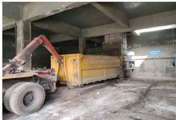
A container connected with hopper at ground floor
