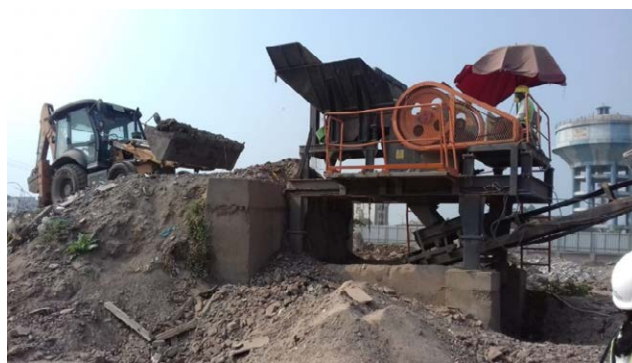
Crushing Machine of C&D Plant
