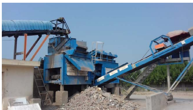
Washing Machine of C&D Plant
