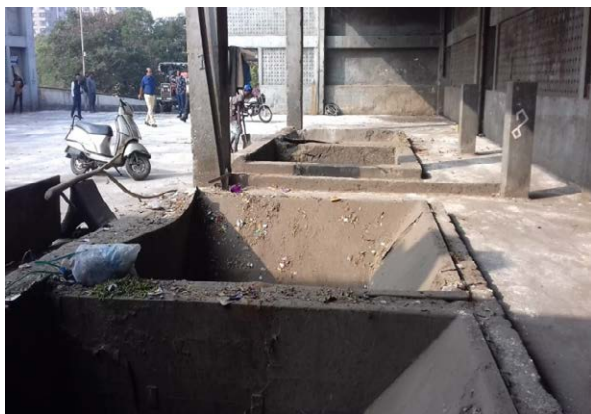
Hopper Chamber at first floor
