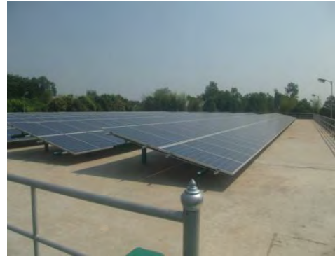
Solar panel at Roof
