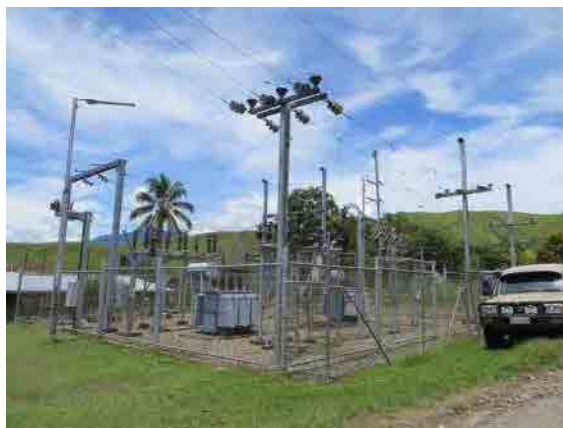
Baiune-1, 33/22kV 変電所全景
