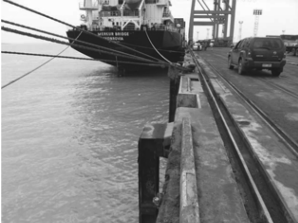
Photo 3.3.12 Fender (at Berth No. 4)
