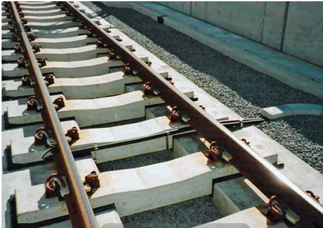
(Remark; the ballast is used not for track, but for reduction of noise) Source; Internet web-site, D-type solid bed track, Nakanoshima Line of Keihan railway
