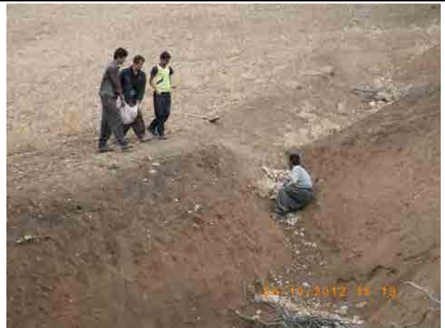
Reinforcement work of check dam which are damaged by snow-melt water in spring. They are carrying bags filled with stones.
