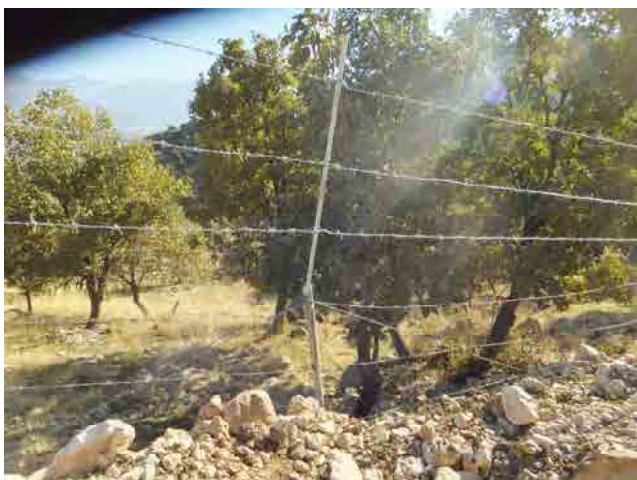
The fence repair situation; the damaged part are inclined with pushing soil with the repair work of the road improvement construction. (October, Tabarak Sofla)
