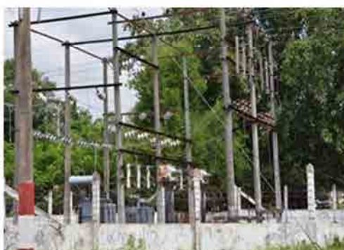
YAU電源供給変圧器1
