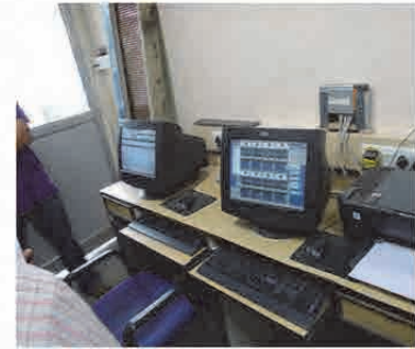
Figure 3-30 City Bus Operations Monitoring Room (Indore)
