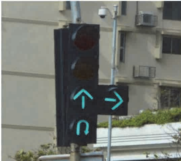
Figure 3-38 Traffic Signal (Mumbai)
