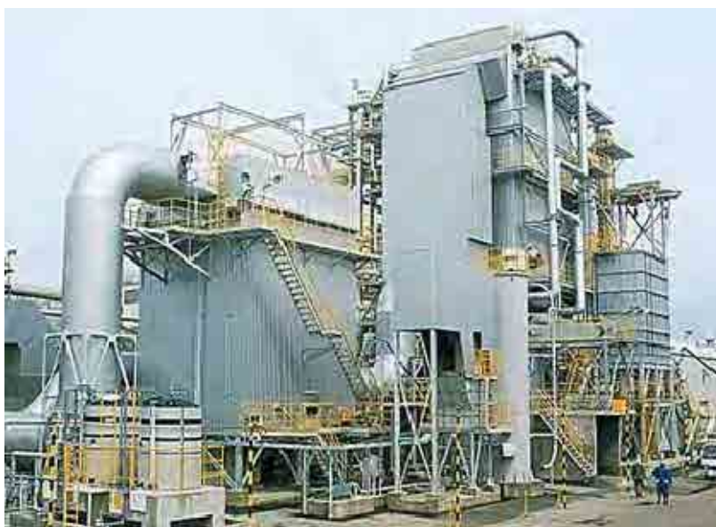
Image 5.1-3 Takuma's Wood Waste-fired Boiler
