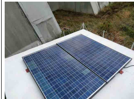
Existing PV Panel
