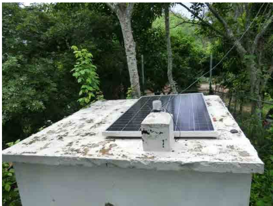
Existing PV Panel
