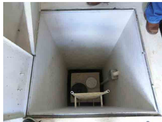
Install position of Broadband Seismometer
