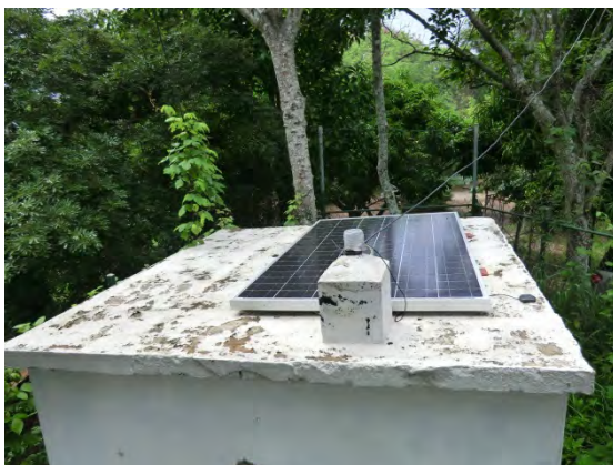
Existing PV Panel
