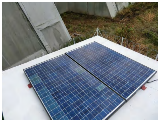
Existing PV Panel
