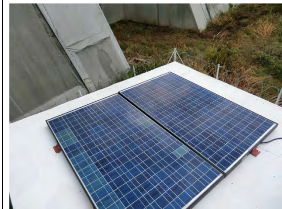
Existing PV Panel
