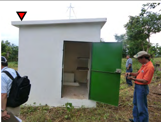
Install position of GPS sensor 2
