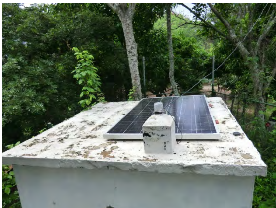
Existing PV Panel
