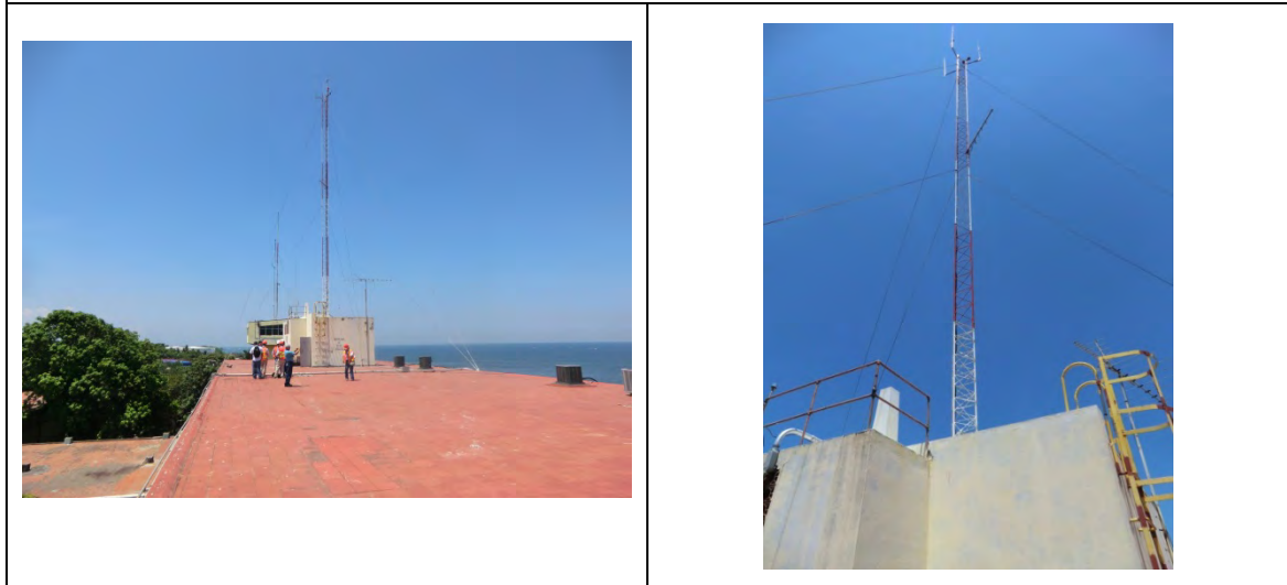
Install area(Top of staircase of CEPA's Building)
