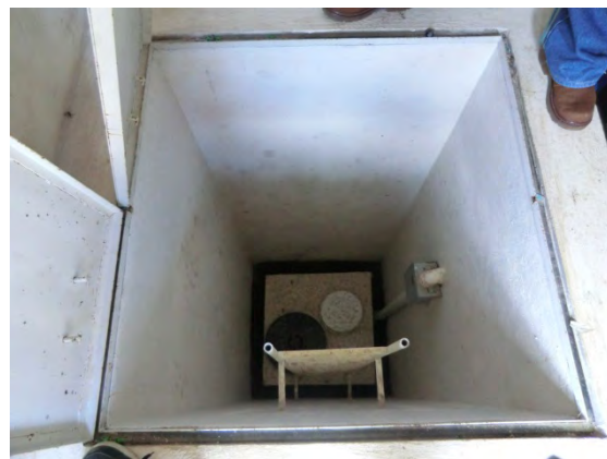
Install position of Broadband Seismometer
