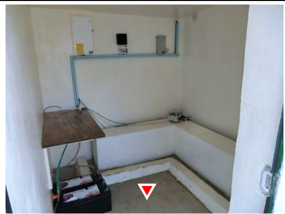
Install Area of Broadband Seismometer
