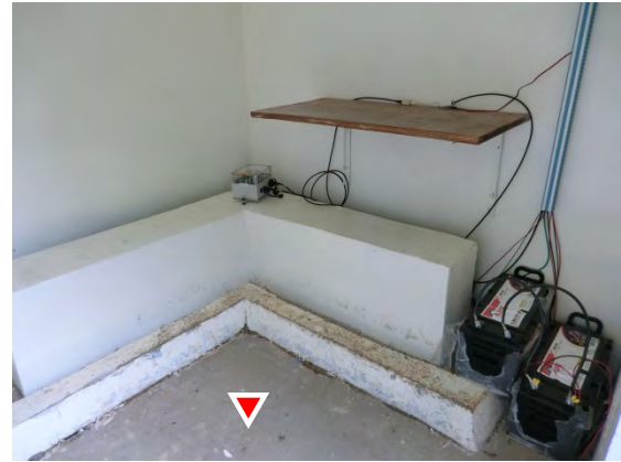
Install Area of Broadband Seismometer
