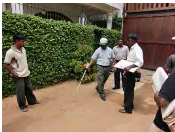
Borella Valve Locating
