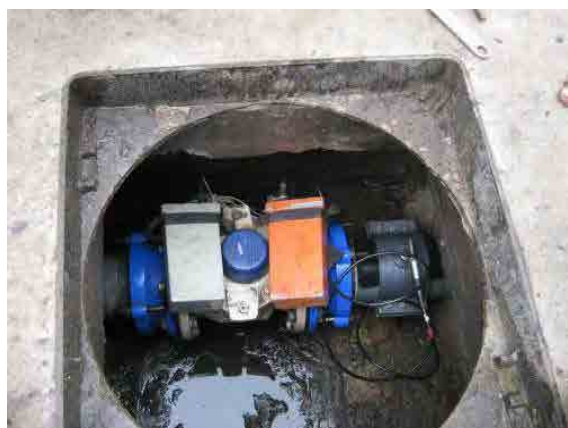
Kotahena Flow Rate Measurement
