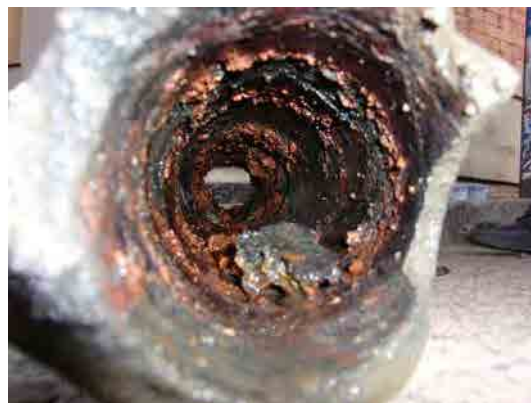
Borella Inner Surface of Old CI Pipe
