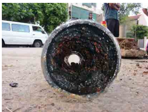
Borella Inner Surface of Old CI Pipe
