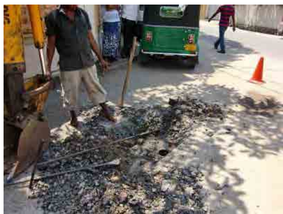
Borella Valve Locating
