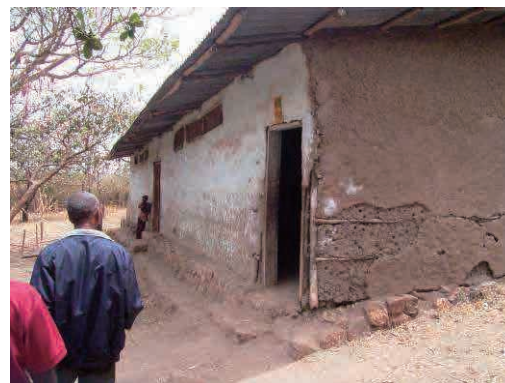
A dilapidated school building
