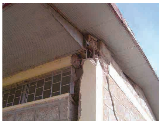
A damaged building by an earthquake <adjacent primary school to the site>
