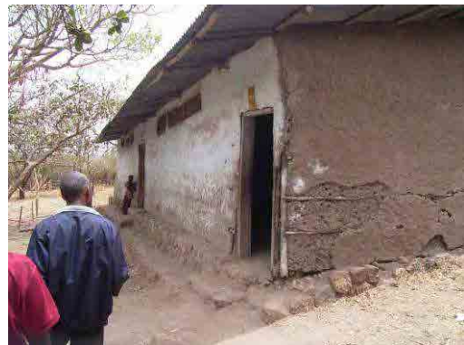
A dilapidated school building
