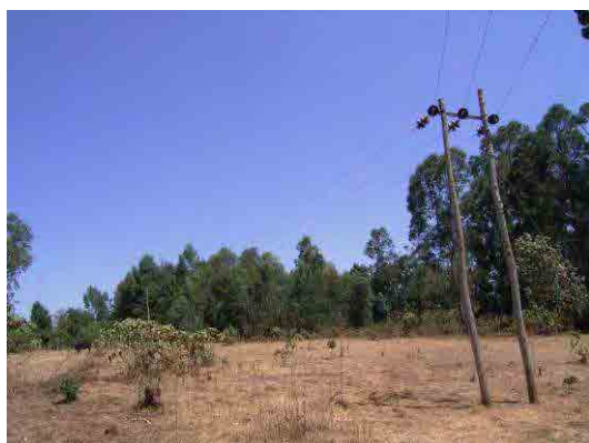
Power lines within the construction site
