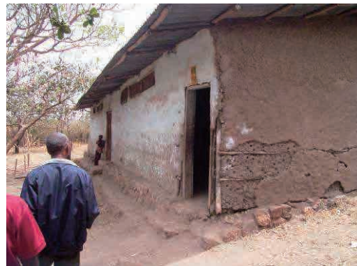
A dilapidated school building
