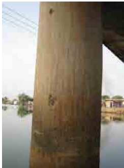
Photo-9 Damage by Shot (P-2)
