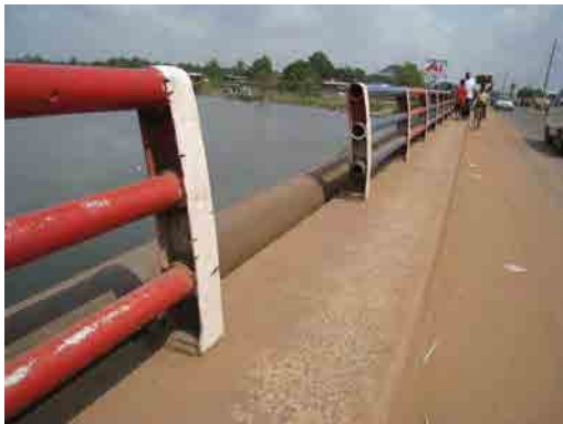
Photo-1 Missing Pipe (Upstream side)
