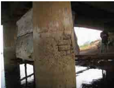
Photo-11 Damage of P-3, Center
