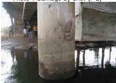
Photo-10 Damage of P-3, Upstream side
