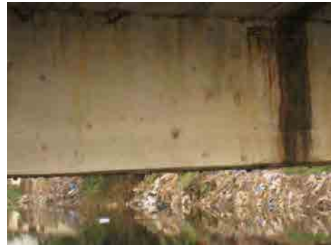
Photo-9 Damages by shot
