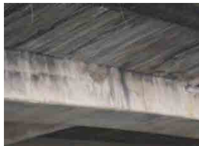
Photo-7 Damage by Shot
