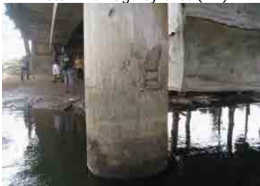
Photo-10 Damage of P-3, Upstream side
