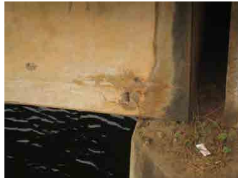
Photo-9 Appearing Reinforcement bar
