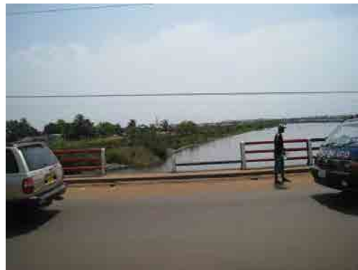
Photo-2 Missing Pipe & Pole (Downstream side)
