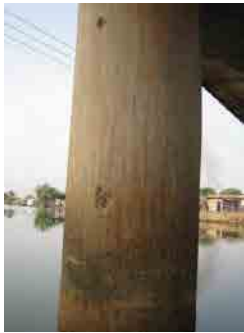
Photo-9 Damage by Shot (P-2)
