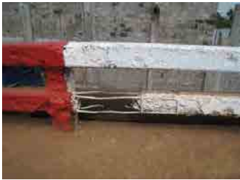
Photo-1 Broken Railing
