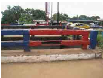
Photo-2 Broken Railing
