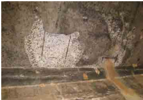
Photo-5 Appearing Reinforcement Bar
