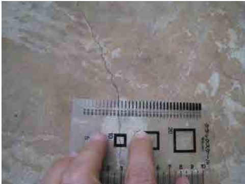
Photo-8 Crack Width (W=0.4mm)
