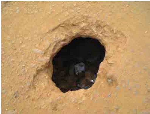
Photo-4 Hole on Slab (D=230mm)
