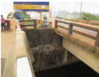
Photo-2 Broken Railing
